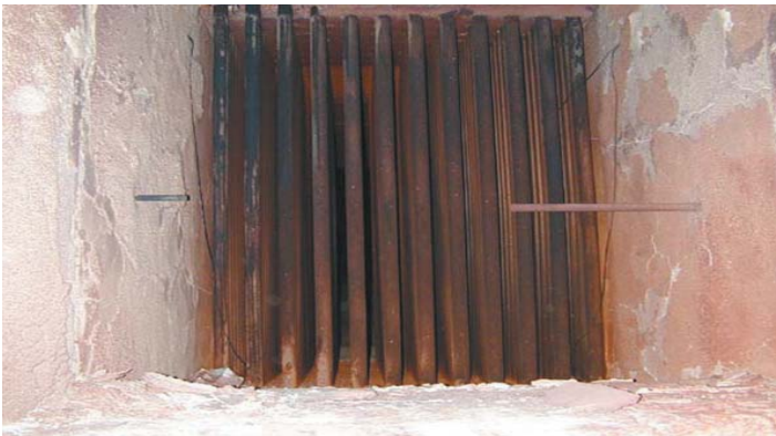
RA 253 MA pipe replaced type 310 stainless steel in this recuperator system off of a zinc galvanizing line. Estimated process temperatures were 1600°F (average) and 1750°F maximum. The recuperator used 2" SCH40 pipe. 310 and 316 stainless pipe used in the front three rows, the inlet for hot exhaust gases, of the recuperator failed from scaling in less than 1 year. RA 253 MA was installed and photos show its condition after 2 years in service. Latest inspection reported no RA 253 MA after four years of service.
